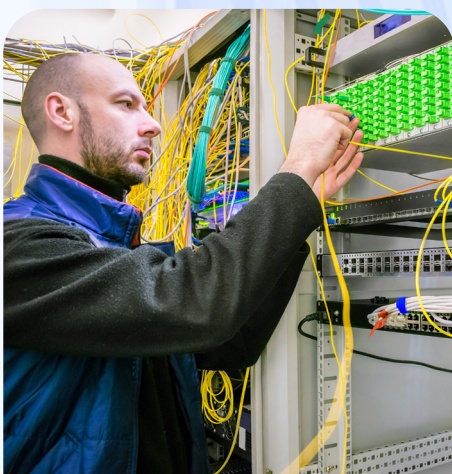
Telecommunication Network Deployment
