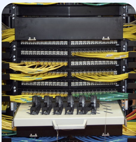
Structured Cabling System
